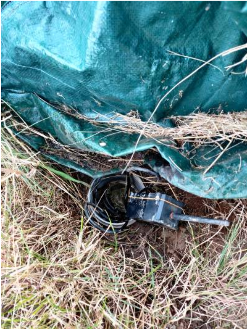
The hole is reinforced with a 15cm long pvc pipe and closed with a lid.
