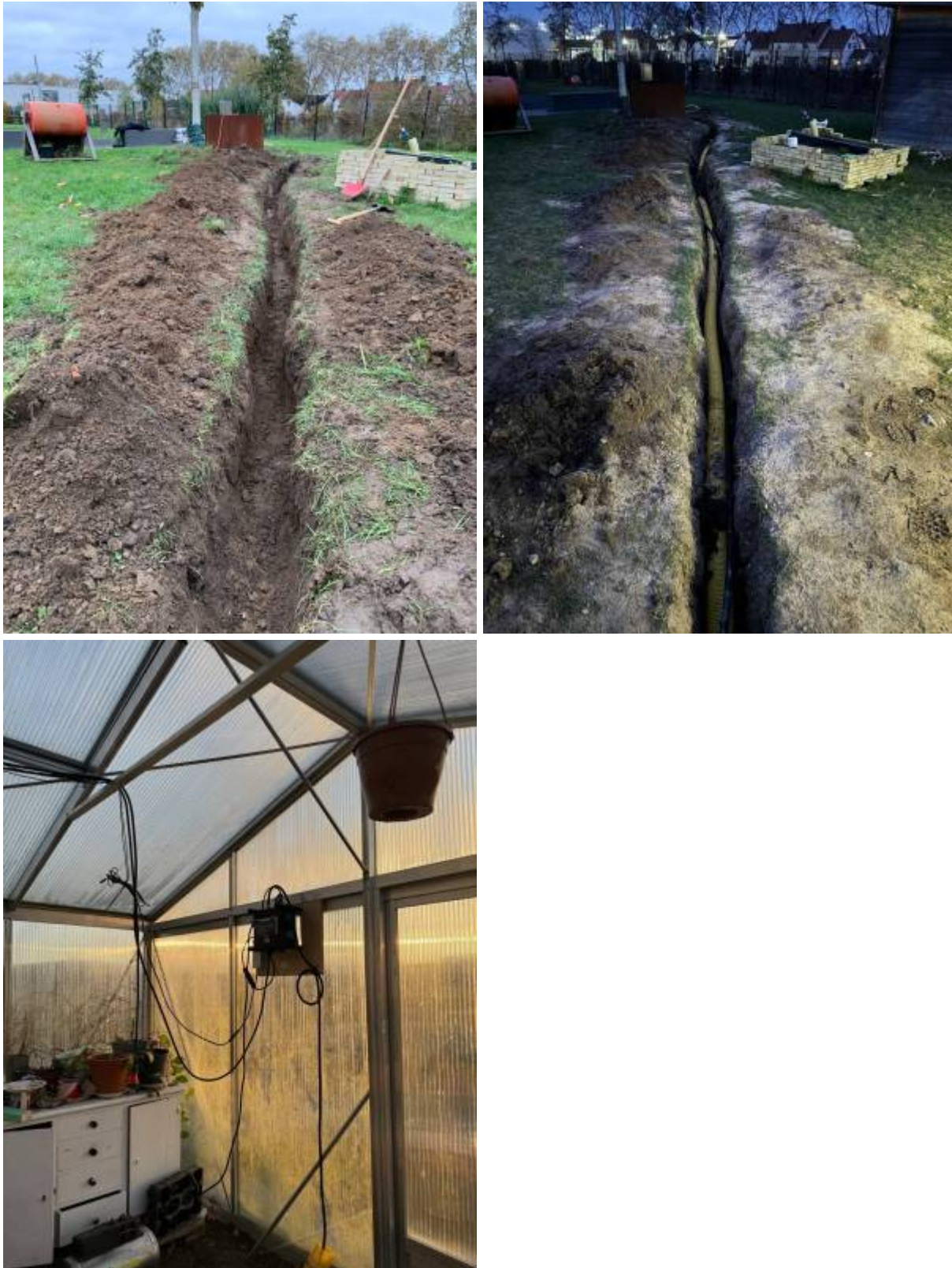
Fig - 8 Pictures of the Trench before the pipe (Left), after the pipe (middle) and the electrical hub (right)
